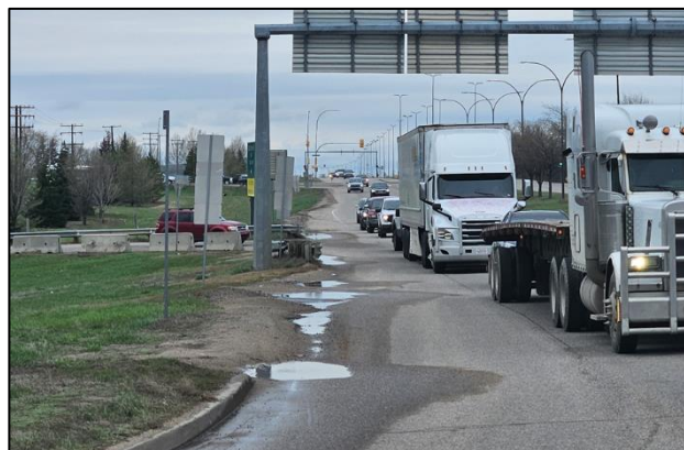
Figure 2-1: Damage to the eastbound shoulder due to vehicles bypassing the vehicle queue
