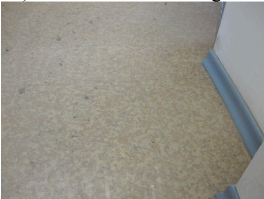
#3) Sheet Floor Covering
