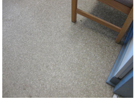
#2) Sheet Floor Covering
