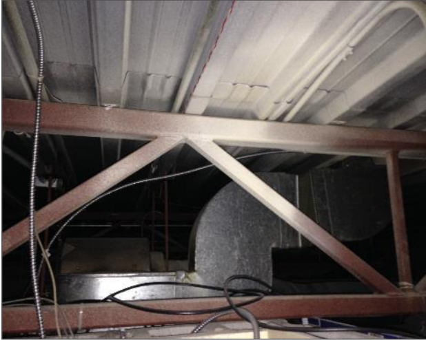
Photo 1: Un-insulated metal duct, structural steel, and metal roof decking above acoustic ceiling tiles in Men's Washroom (Location 105)
