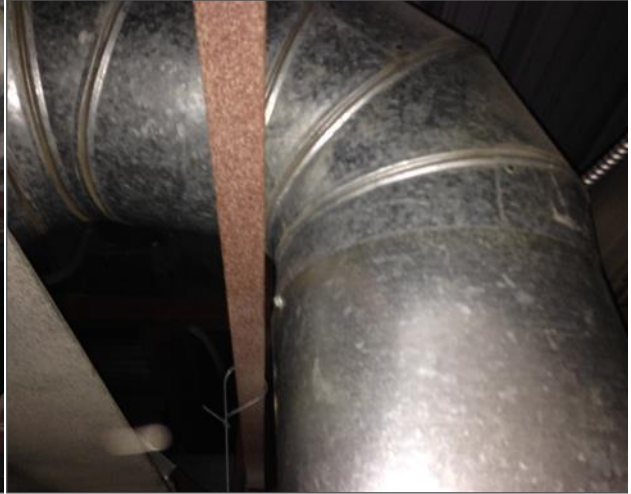
Photo 2: Un-insulated metal duct with no mastic above acoustic ceiling tiles in Men's Washroom (Location 105).
