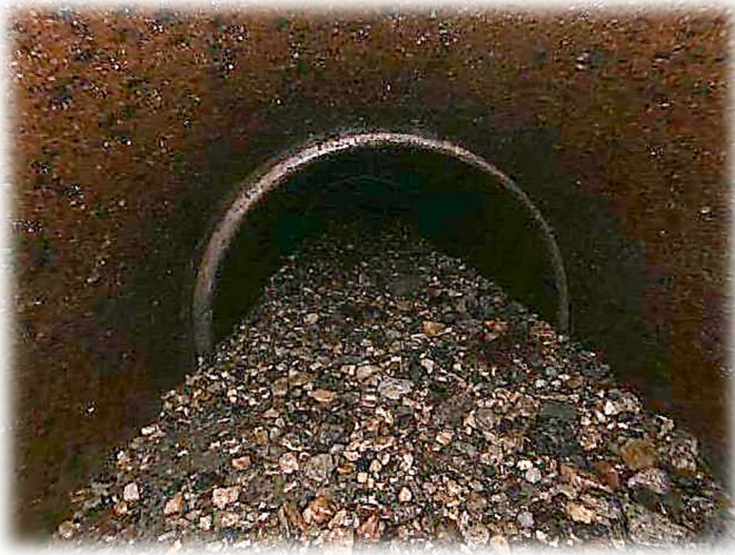
Figure 9: Image of Sediment within Storm Sewer Pipe
