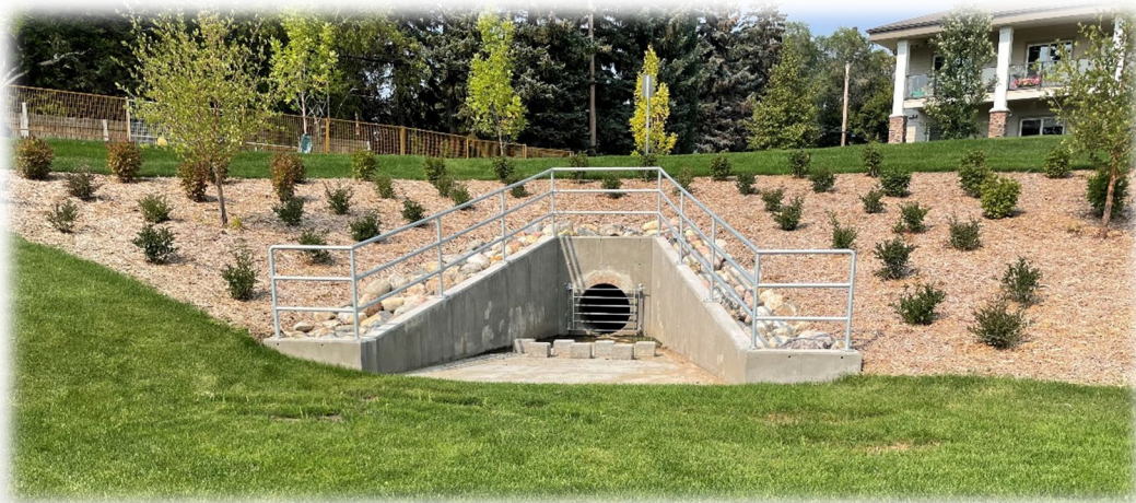
Figure 1: Storm Water Inlet/Outlet Structure in Churchill Park Dry Pond
