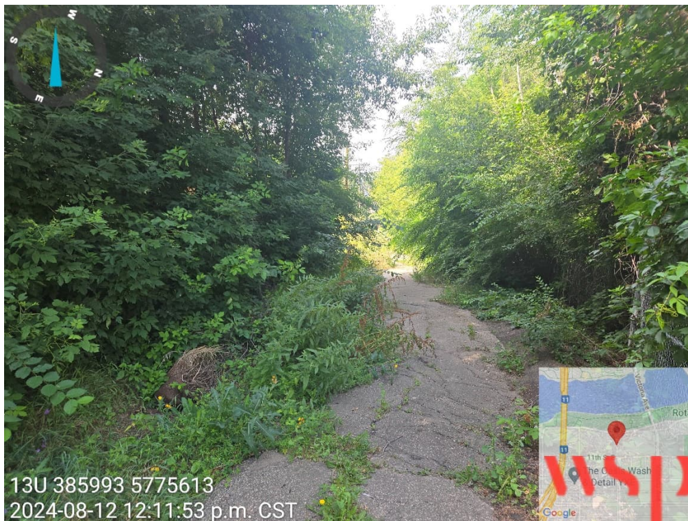
Photograph 2: Looking west down the back alley at the West Failure (August 12, 2024)
