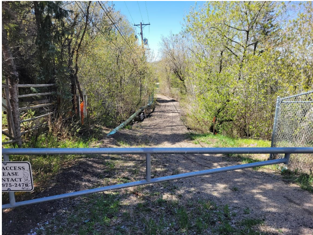
Photograph 1: Looking west down the back alley at the East Failure (May 8, 2024)
