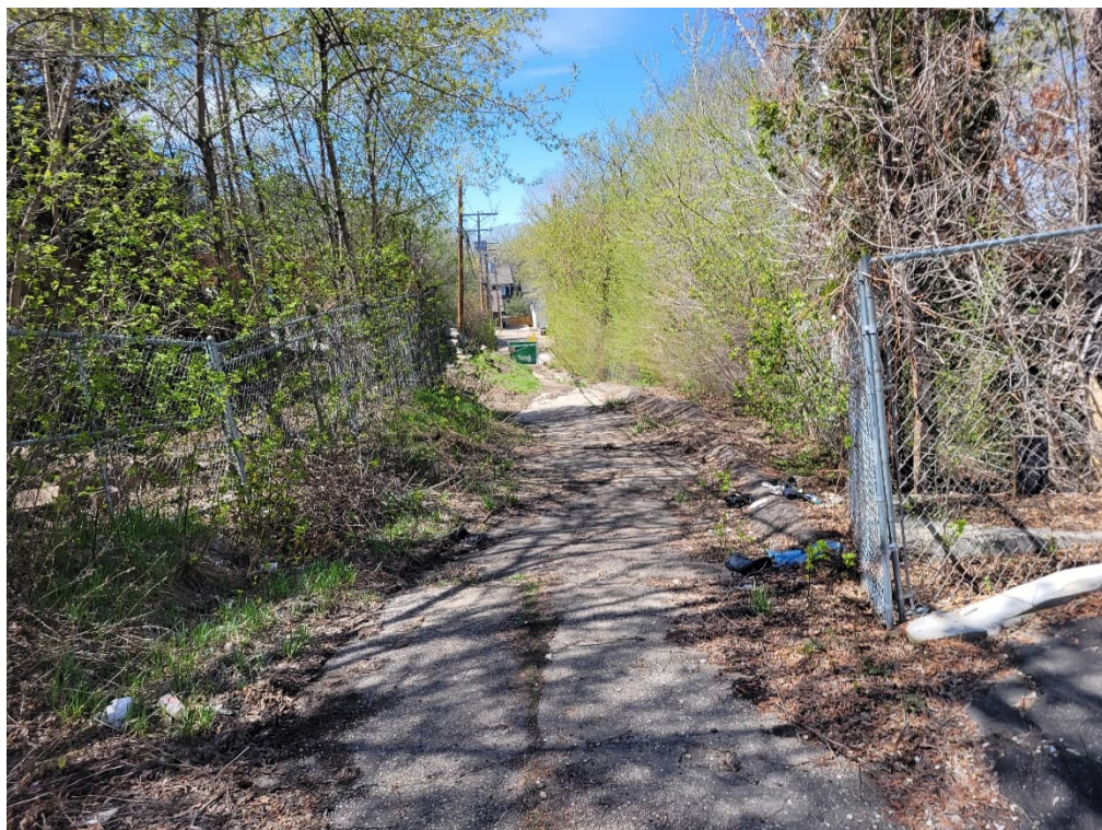
Photograph 2: Looking west down the back alley at the West Failure (May 8, 2024)
