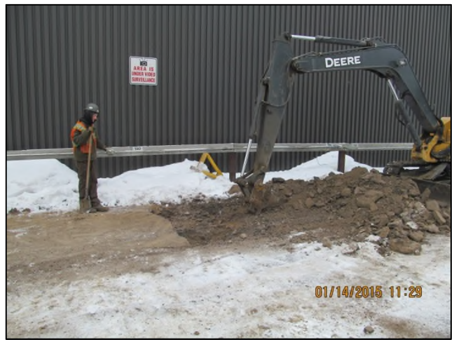
Photo 2: The excavation site. Note the concrete slab uncovered on the eastern portion of the excavation.
