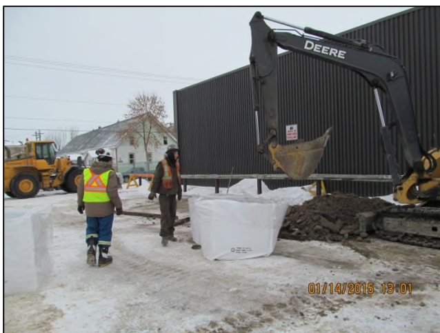
Photo 5: Soil from the excavation being loaded into soil bags for onsite storage.
