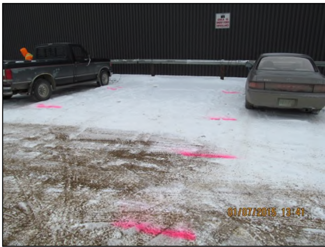
Photo 1: View of the excavation site, looking south. Note the lines indicating the location of historical trolley tracks.
