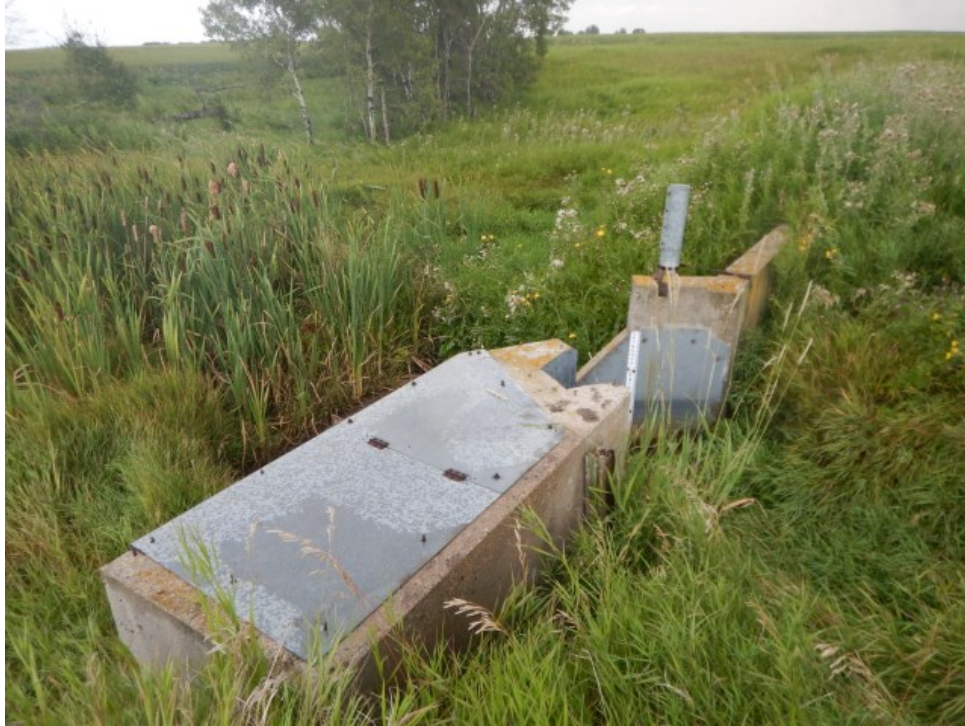
Photo 23: Looking at a water control structure in wetland NW 15-36-04-002 from within the wetland basin on August 11, 2015.
