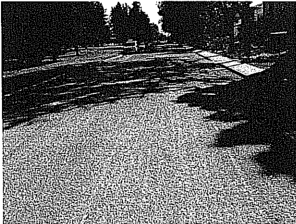
1100 blk Colony prior to seeping – 2006
