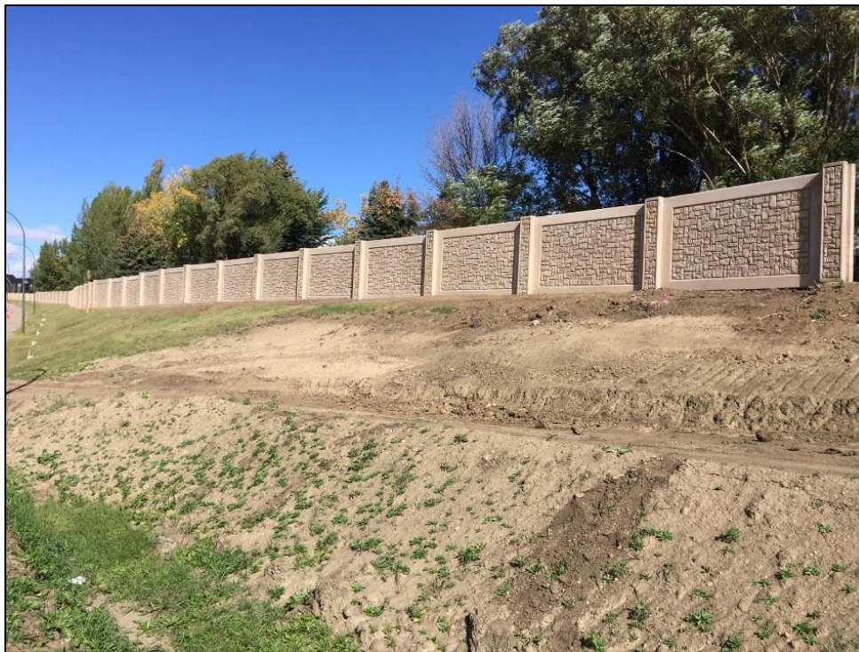
Stone tree fence installed at north end of Lakeview location (before final grading/seeding).
