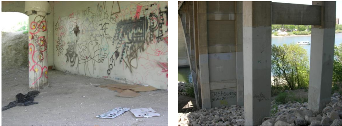
Above: Examples of the Broadway Bridge victimized by graffiti vandalism.
