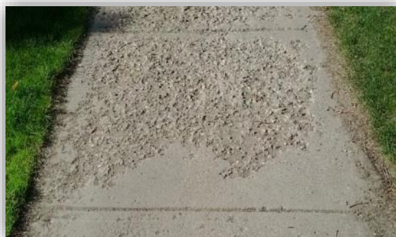
High Severity – Replacement
