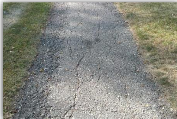
Fair Condition Asphalt Overlay Replacement or Overlay/Seal
