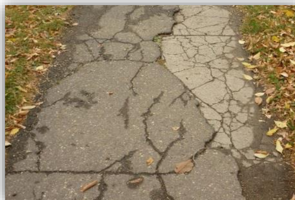
Poor Condition Asphalt Overlay Replacement
