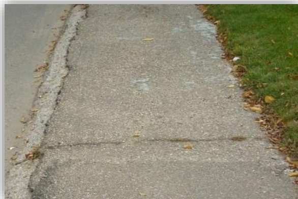
Good Condition Asphalt Overlay Curb Deteriorated - Replacement
