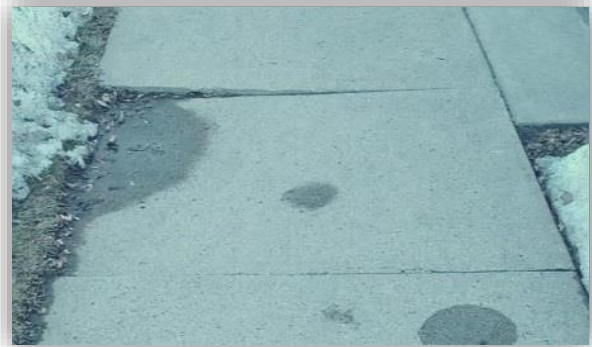
Mud Jack or Replacement
