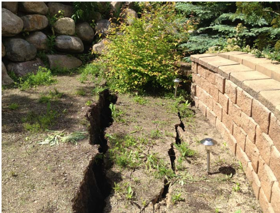
Photo C.8. Cracking Behind Retaining Wall in Backyard of 237-239 11th St. E. (June 21, 2012)
