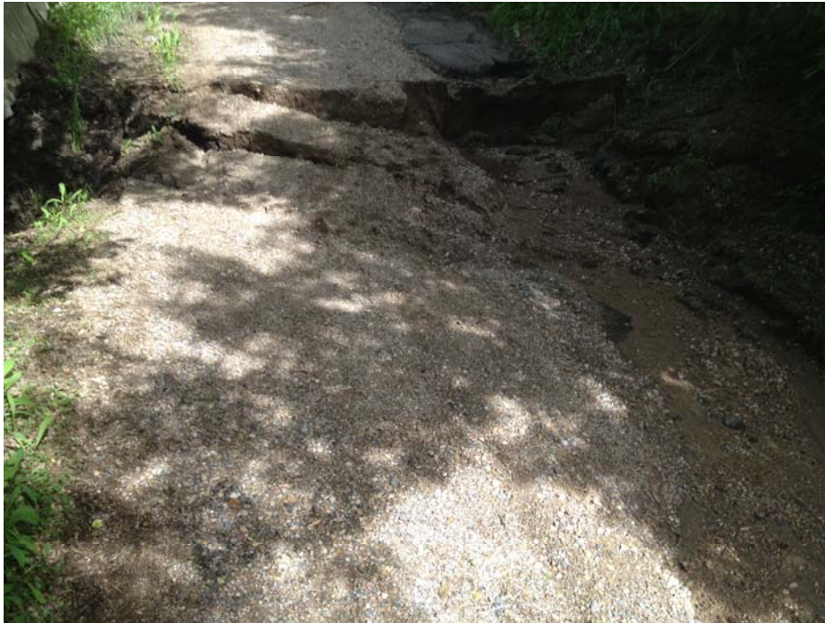
Photo C.15. Looking East at Severe Cracking across Cherry Lane, Pavement; Approx. 50 cm Drop (June 24, 2013)
