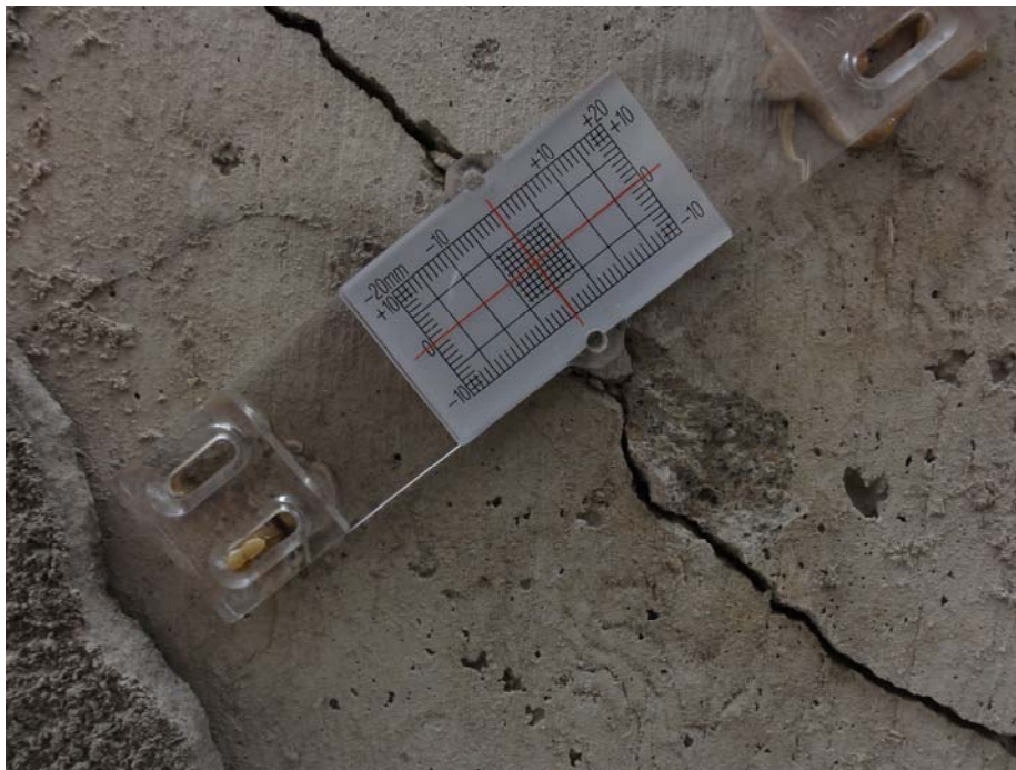
Photo F.6: Crack Meter Located on the West Face of the Retaining Wall Between 230 & 306 Sask. Cres. E. (CM3) (Sept 18, 2013)
