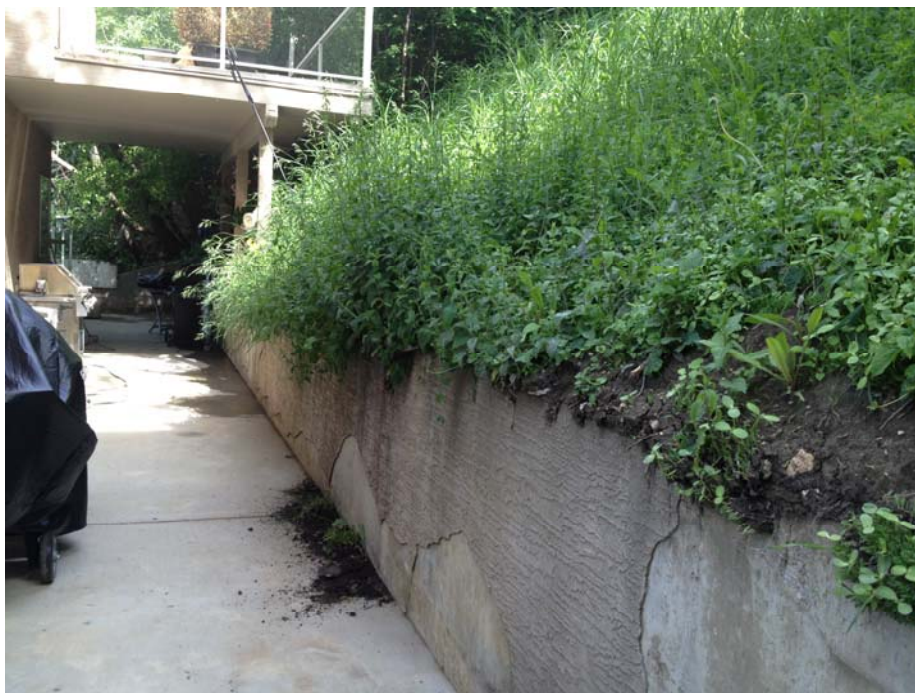
Photo C.14. Looking East at Bulging Toe of Slide above Retaining Wall behind 306 Sask. Cres. E. (June 24, 2013)
