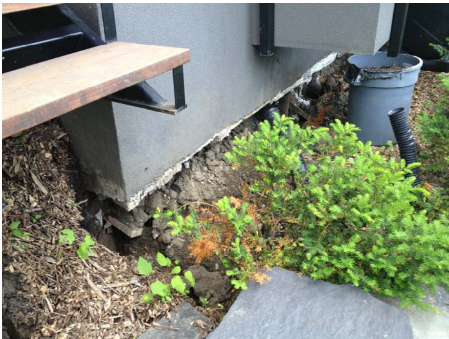
Photo C.13. Headscarp of East Failure in Backyard of 303 11th St. E.; Approx. 60 cm Drop (June 24, 2013)
