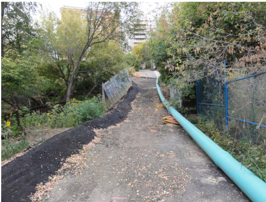
Photo C.29. Looking East at Above Ground Driantage System Installed on Cherry Lane (September 18, 2013)
