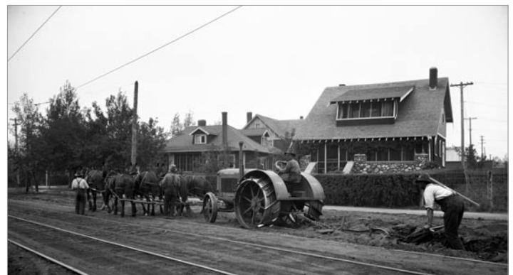
Plowing a trench on Avenue E North near Bedford Road with the two-storey house, 511 Avenue E North, in the background, c. 1920 [Leonard A. Hillyard photo] (Saskatoon Public Library Local History Room A-2542)
