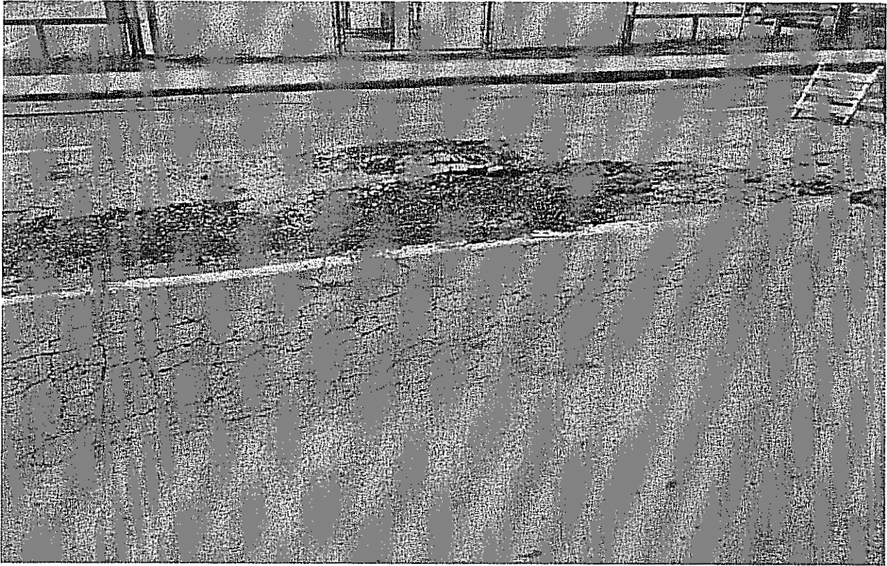
Figure 5: Fairlight Drive – McCormack Road to 11 th Street West (Estimated Repair Cost $91,000)
