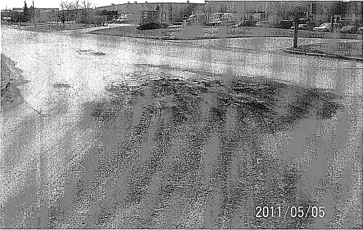
Figure 4: Thatcher Avenue approaching 71 st Street (Estimated Repair Cost $320,000)
