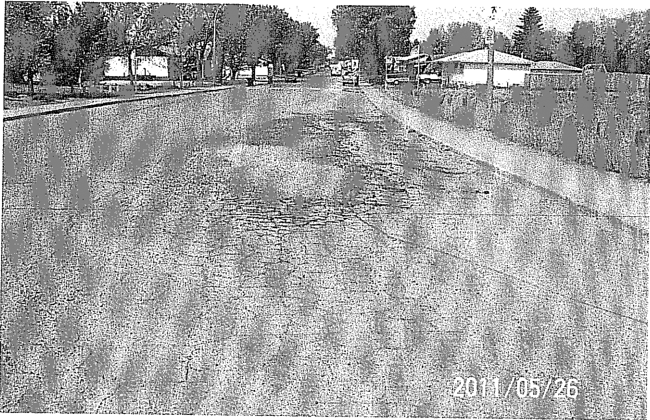
Figure 3: 37 th Street – Avenue W to Byers Crescent (Estimated Repair Cost $70,000)
