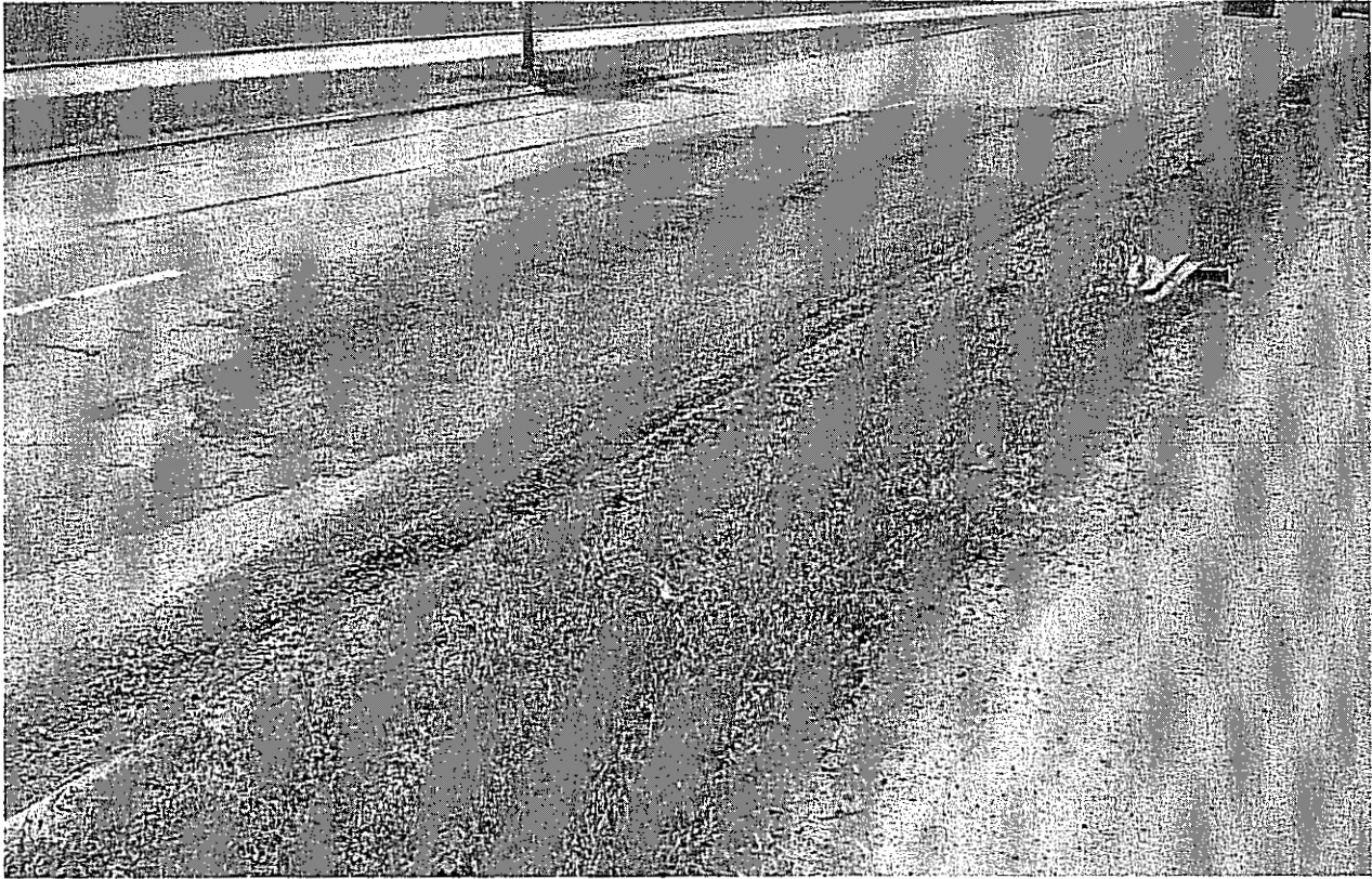
Figure 1: Attridge Drive from Lowe Road to Nelson Crescent (Estimated Repair Cost $568,000)
