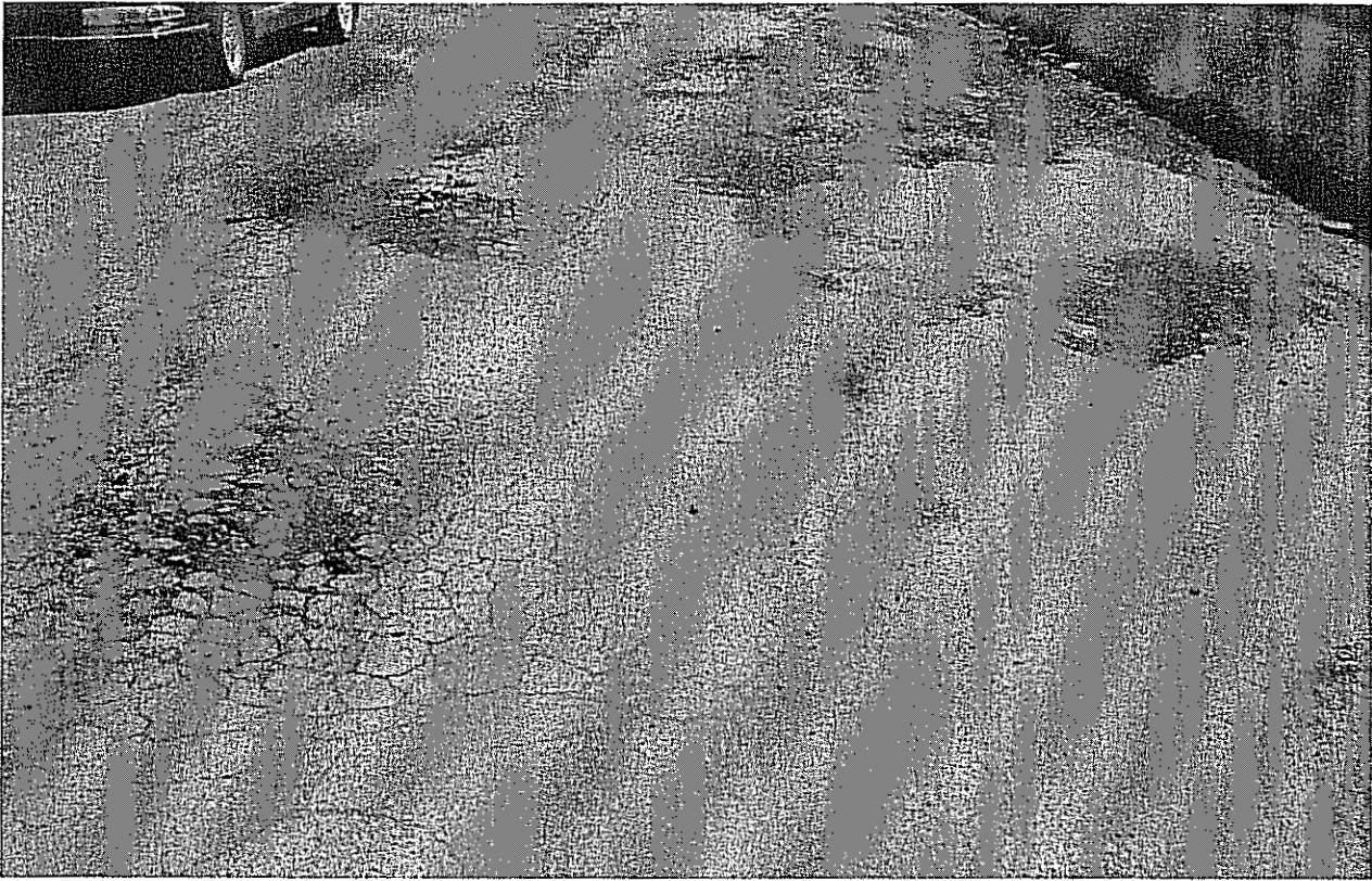
Figure 2: Duchess Street – 6 th Avenue to 7 th Avenue (Estimated Repair Cost $108,000)
