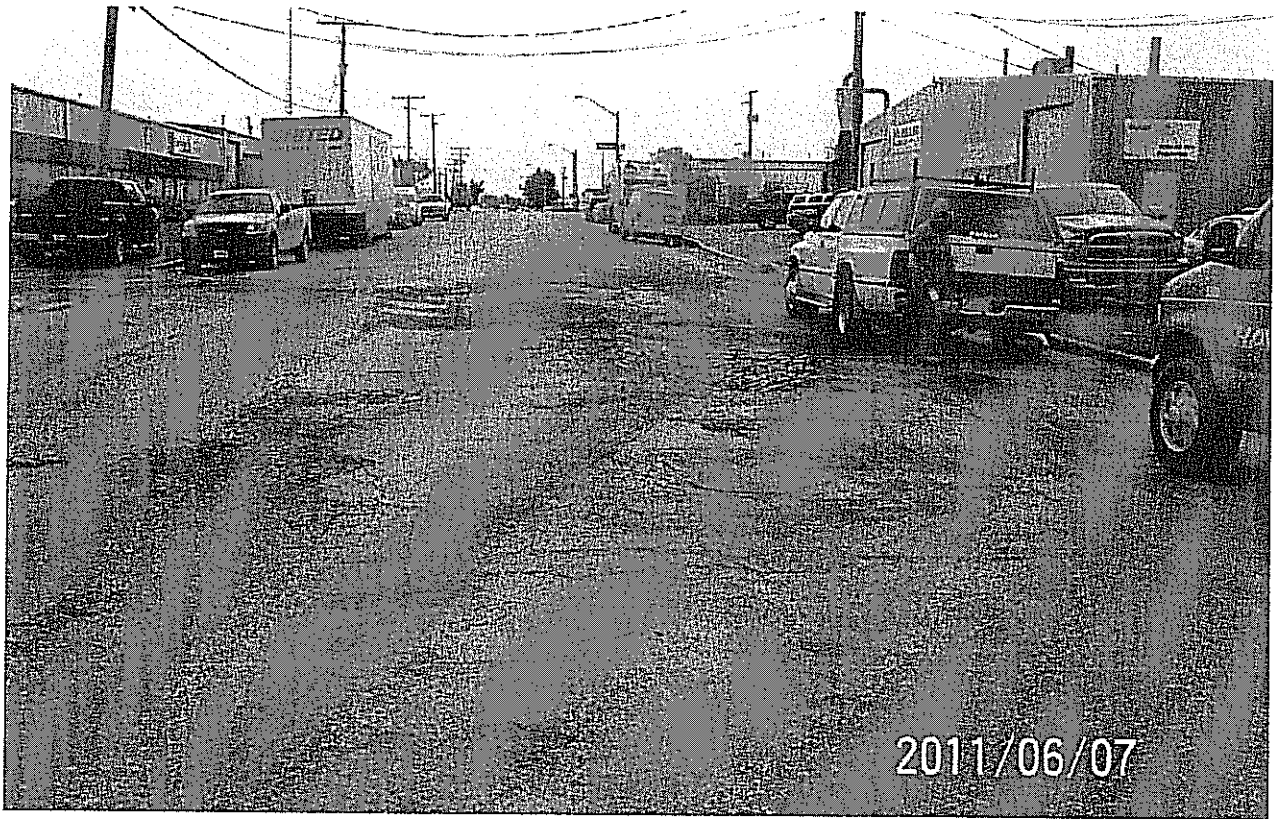
Figure 6: 47 th Street – Faithfull Avenue to 1 st Avenue (Estimated Repair Cost $180,000)
