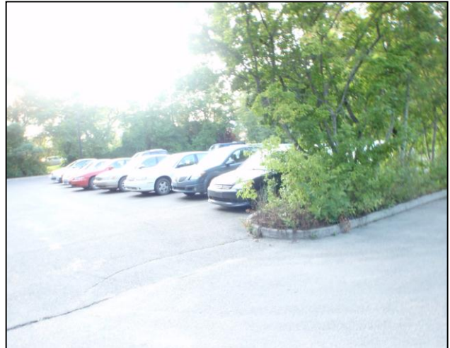
Surface pavement cracks and depressions.
