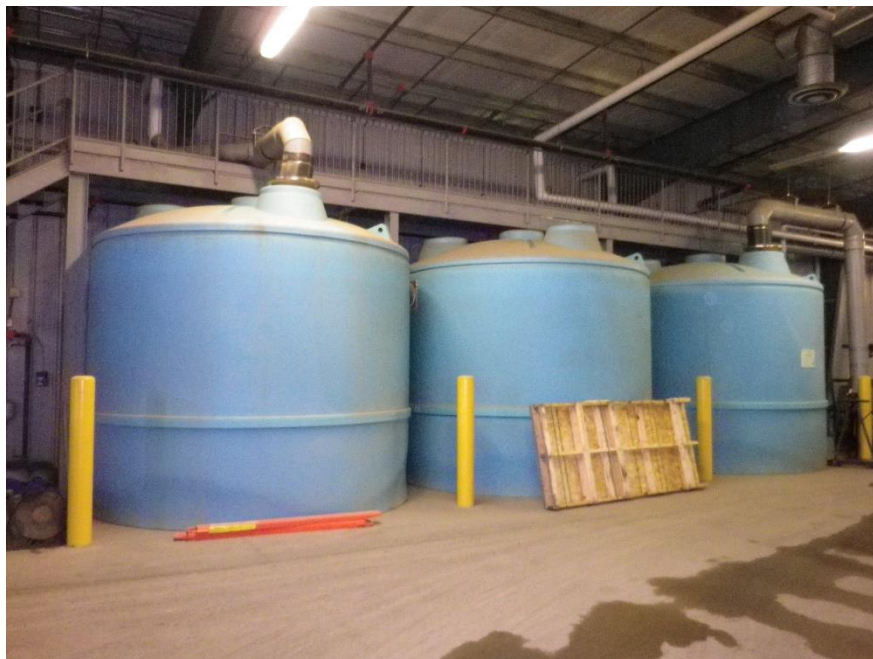
Figure 27: 35,000 L Tanks at Access Transit Garage, Saskatoon
