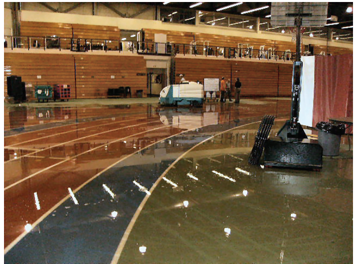
Saskatoon Field House Flood, June 30 th , 2010
