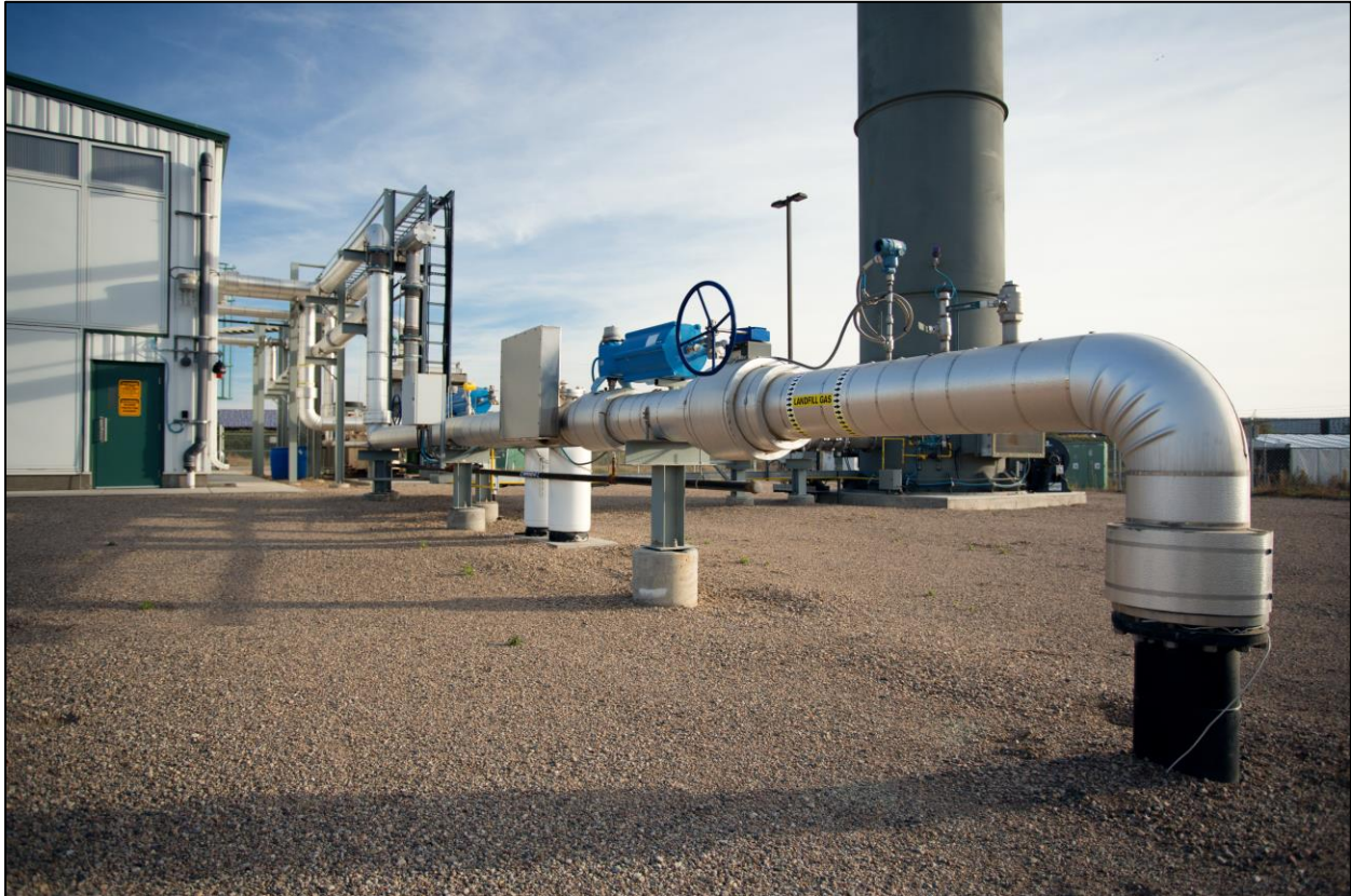
Landfill Gas Collection and Power Generation Facility
