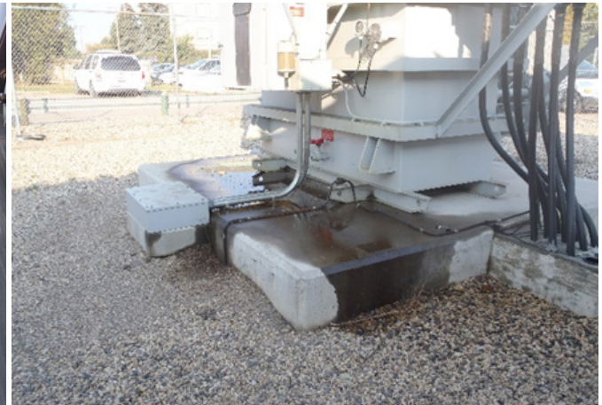
Substation Transformer Oil Leak (College Park)
