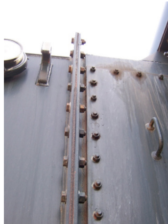
Substation Transformer Oil Leak (1st Ave)
