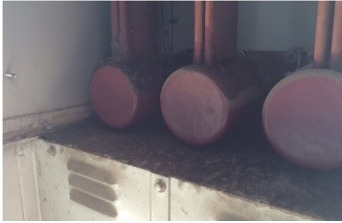
Dirt and Contamination Inside Switchgear
