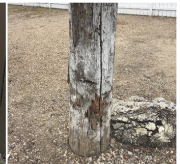
Wood Distribution Pole - Poor Condition
