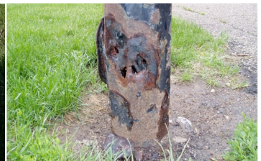
Street Light Pole in Poor Condition
