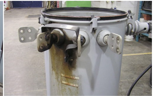
Leaking Overhead Distribution Transformer
