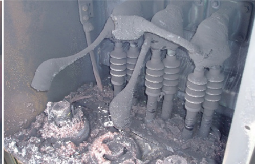
Switchgear Failure from Contamination
