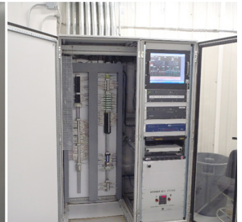
Substation Control Cabinet
