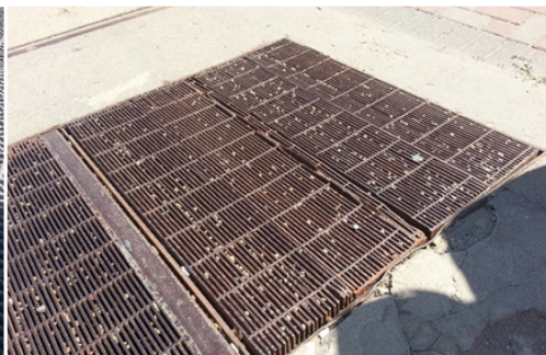
Network Vault Grate in Poor Condition
