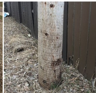
Wood Distribution Pole - Good Condition
