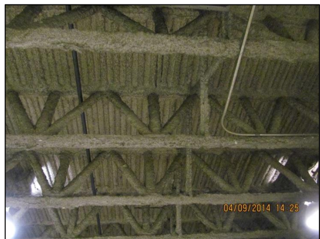
Photo 12: Blown-on fire retardant insulation, likely a form of cellulose, ceiling of bus storage barn, 301 24 th Street W.
