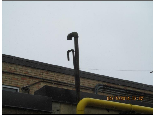
Photo 20: Vent lines in southwest loading area, adjacent to boiler room exterior wall, at 321 Ave C N looking west.
