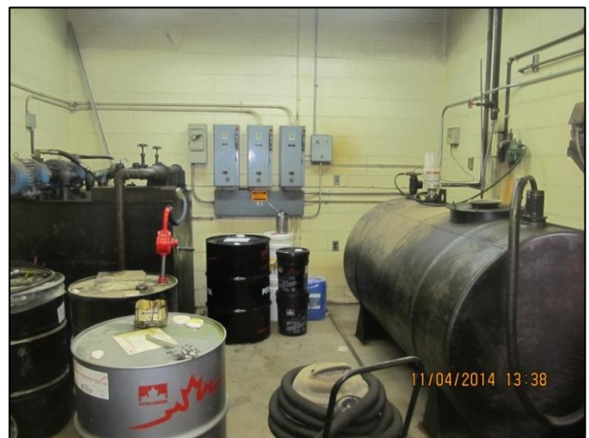
Photo 34: The fluid distribution room in the southeast corner of Shop B at 321 Ave C N.
