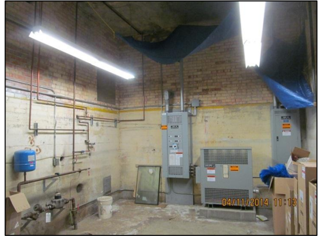
Photo 26: The boiler room at 321 Ave C N. Note the electrical transformer and concrete patch on the floor.
