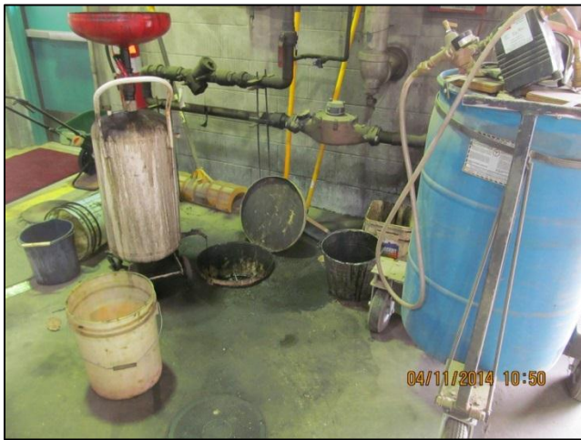
Photo 21: Used oil interceptor in northeast corner of maintenance shop at 301 Ave C N.
