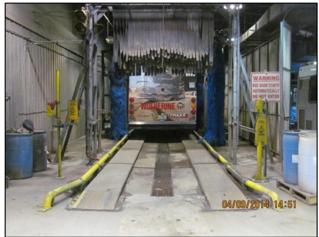
Photo 10: The bus wash, bus storage barn, 301 24 th Street W. Note chemical storage drums and drainage grate.
