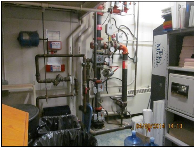
Photo 7: Mechanical room, 301 24 th Street W. Note fire suppression system.
