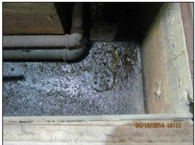
Photo 24: Piping for hydraulic hoists in maintenance garage at 301 Ave C N looking. Note the oily sludge and drain.
