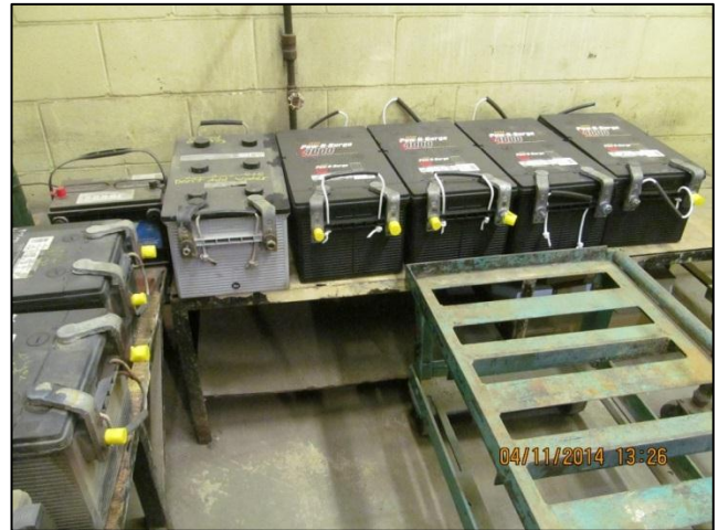
Photo 32: Automotive batteries in the battery room located adjacent to Shop B at 321 Ave C N.
