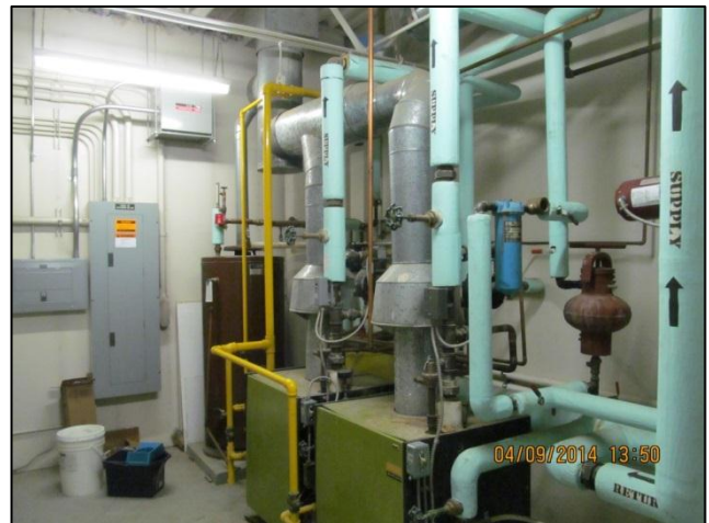
Photo 6: Mechanical room, 301 24 th Street W. Note pipe wrap elbows as potential source of asbestos.
