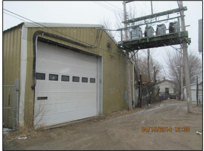
Photo 44: Platform mounted transformers adjacent to southeast corner of 316 Ave C N.
