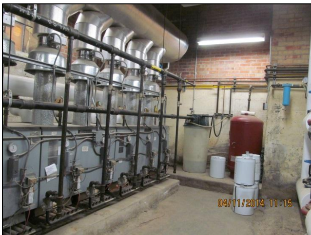
Photo 27: The boiler room at 321 Ave C N. Note exterior buildings materials.
