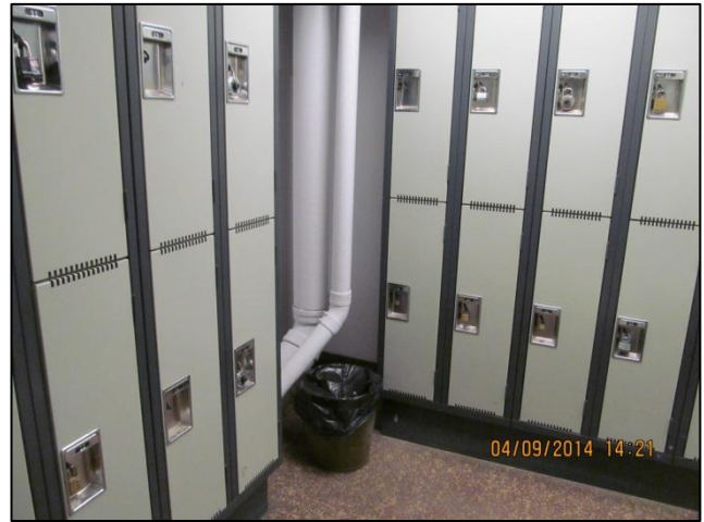
Photo 8: Men's locker room, 301 24 th Street W. Note sewer pipe wrap as potential source of asbestos.
