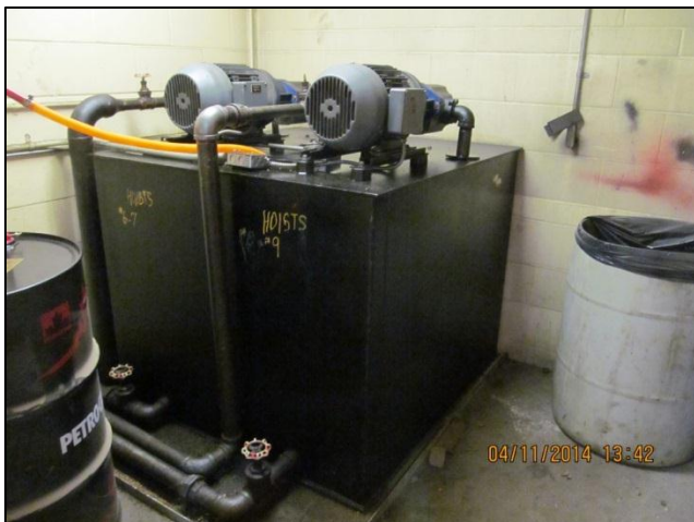
Photo 35: The fluid distribution room located in the northeast portion of Shop B at 321 Ave C N.
