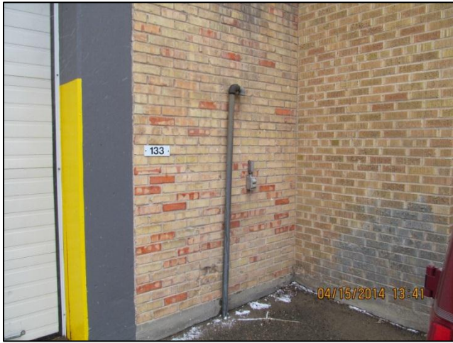
Photo 19: Vent line in southwest loading area, adjacent to boiler room exterior wall, at 321 Ave C N looking northwest.
