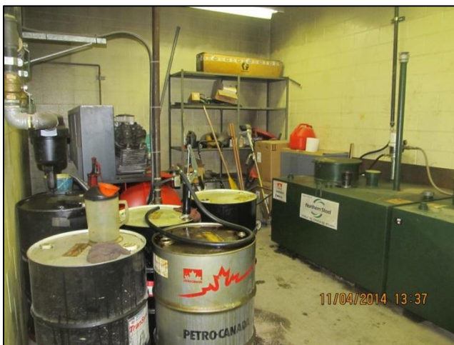
Photo 33: The fluid distribution room in the southeast corner of Shop B at 321 Ave C N.
