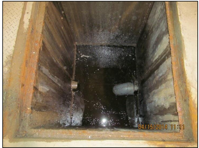
Photo 14: Interceptor sump located in the northeast corner of the bus storage barn, 301 24 th Street W.
