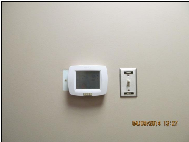
Photo 5: Thermostat mounted on wall, 2 nd floor administration, 301 24 th Street W.
