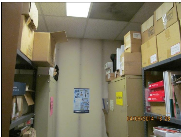
Photo 3: Diesel fume staining in storage area, 2 nd floor administration, 301 24 th Street W.
