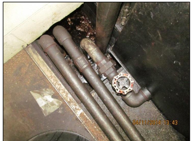
Photo 36: The fluid reservoir in the fluid distribution room located in the northeast portion of Shop B at 321 Ave C N.
