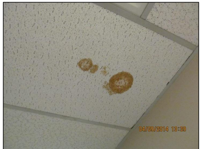
Photo 4: Water stained ceiling tile, 2 nd floor administration, 301 24 th Street W.
