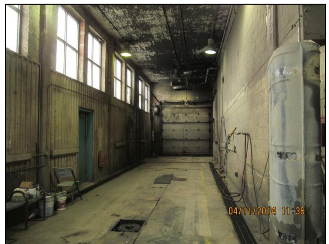
Photo 28: The steam bay in the southwest corner of 321 Ave C N. Note the retired hoist and surficial staining.
