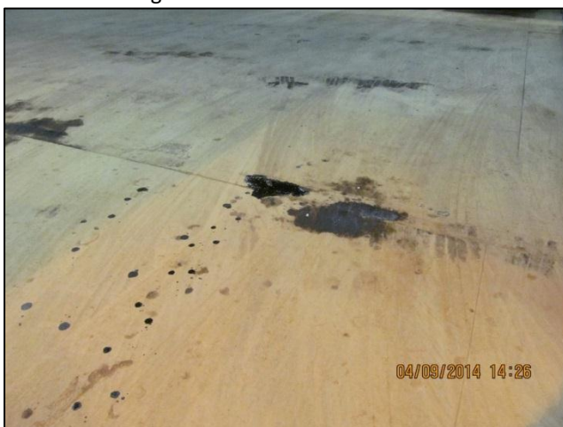
Photo 11: Surficial staining on floor of bus storage barn, 301 24 th Street W.
