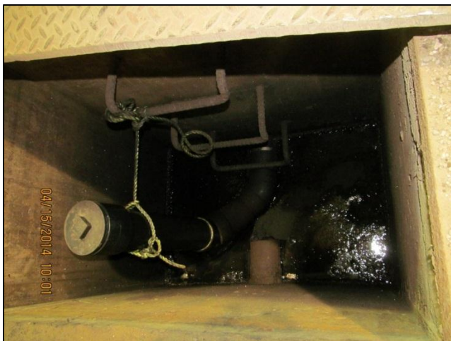
Photo 23: Containment sump located in southeast corner of maintenance garage at 301 Ave C N.
