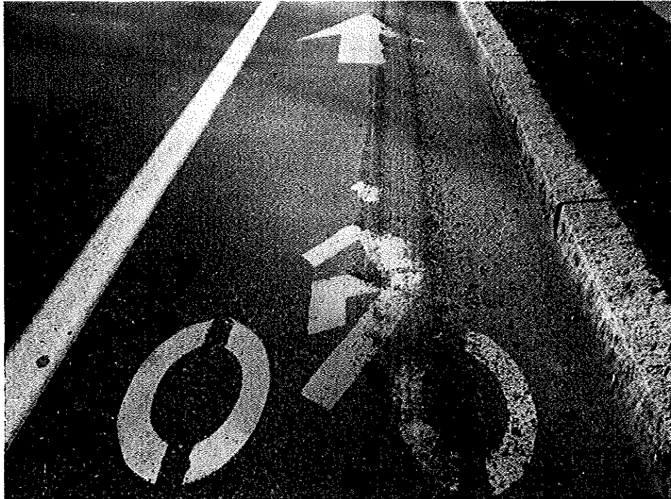
Example: Gravel and sand build up in bike lane – traffic lane is clear.
