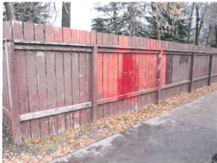
Figure 12: Evidence of Graffiti Vandalism
