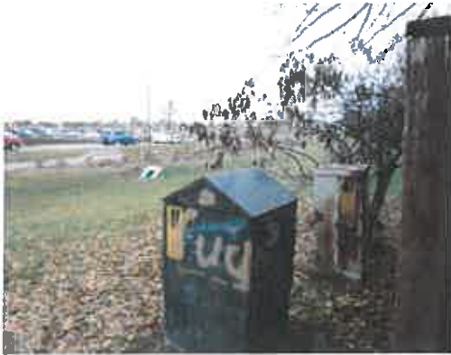
Figure 7: Evidence of Graffiti Vandalism
