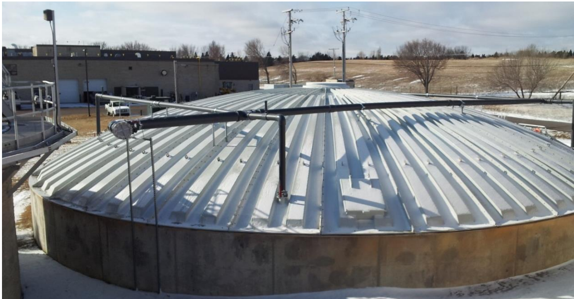
Waste Activated Sludge Stripping to Remove Internal Phosphorous (WASSTRIP) Tank with cover to reduce odour
