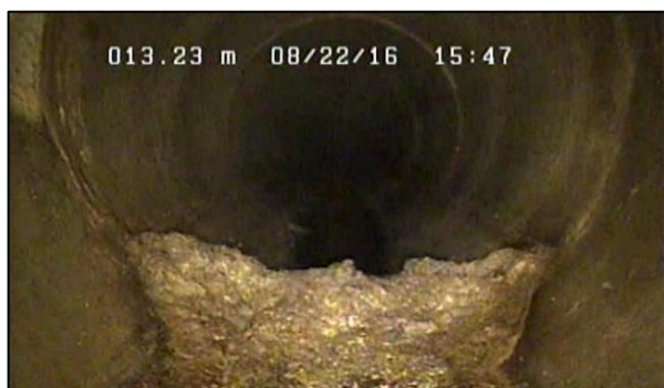
Camera Inspection of storm water pipe showing partial blockage
