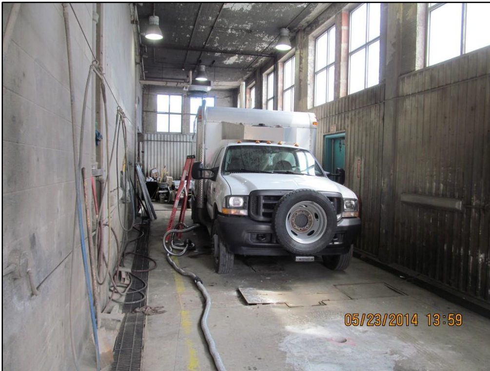
Photograph #9: Steam Bay, located in maintenance building at 321 Avenue C North. Borehole 14-31 is located behind the drill rig.
