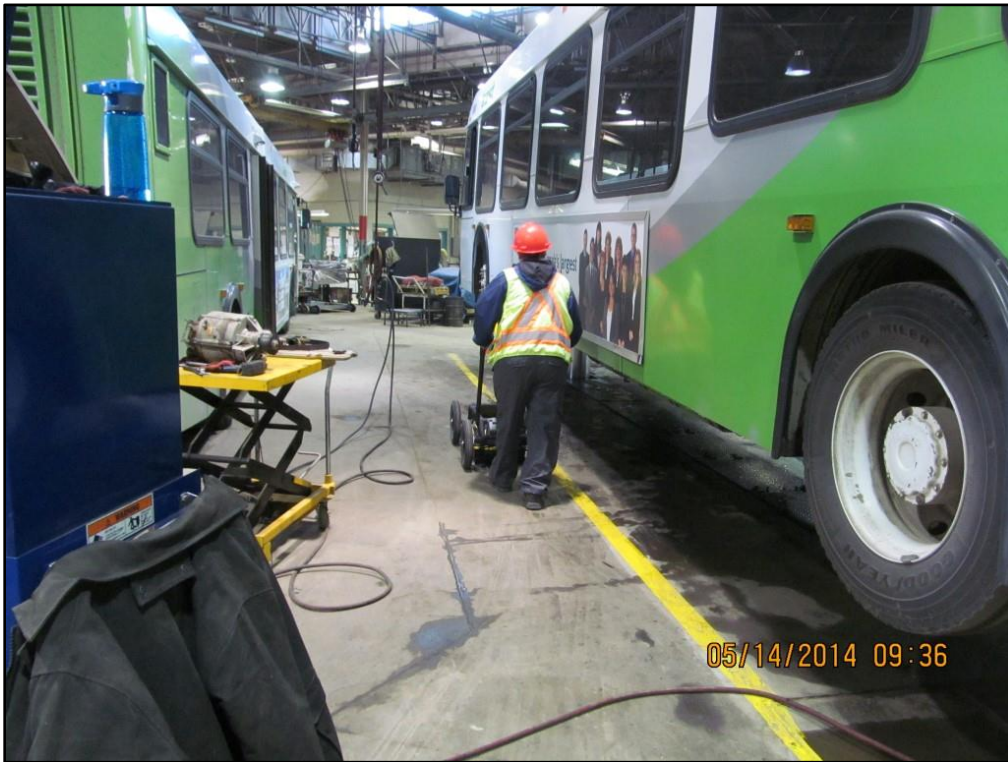
Photograph #1: Ground penetrating radar (GPR) in maintenance shop at 321 Avenue C North.
