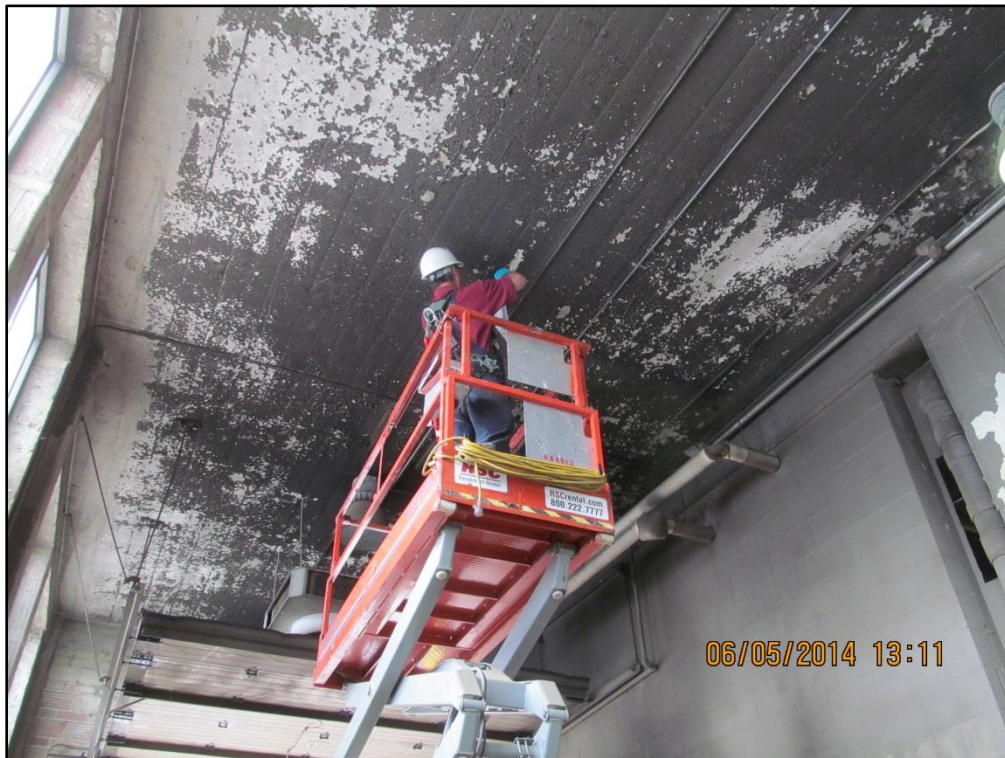
Photograph #12: Sampling for lead-based paint, Steam Bay, maintenance shop located at 321 Avenue C North.
