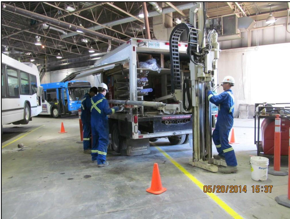
Photograph #6: Advancing borehole 14-8 in the maintenance shop located at 321 Avenue C North.
