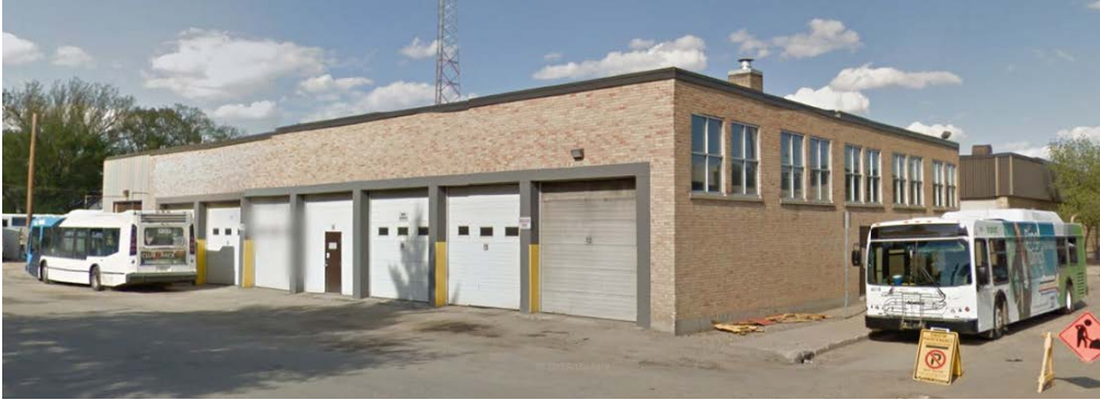
Parcel C – 1948 Building: In good condition; minimal work required to enable reuse.
